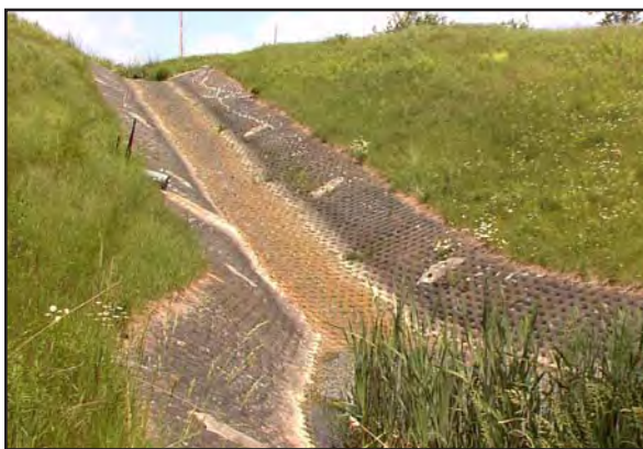
The Stewart Gully erosion control project, erected in 1981, is shown above during a recent inspection.
