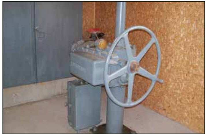
Gate controller for Parkhill Dam.
