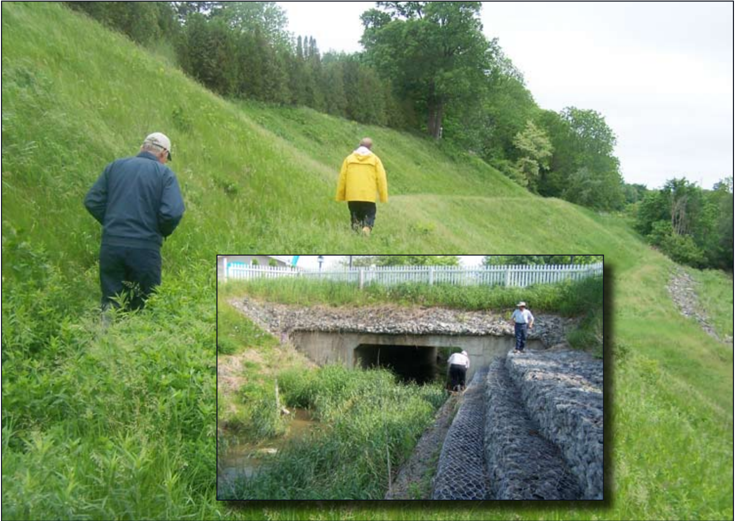
Water and erosion control structures were inspected by Ausable Bayfield Conservation Authority staff in 2007.
