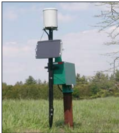
PGMN rain gauge installed in 2007.
