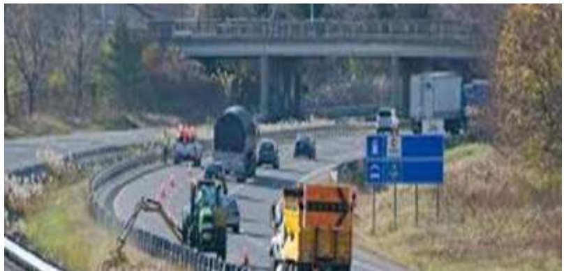
Figure 12. Steve Ford (Green Stream) controlling Phragmites on a section of Highway 403 using WetBlade™ equipment.
